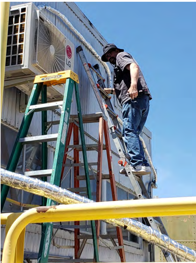
Eric McKay, Don Nelson and Eugene Vicknair teamed up on finishing the new A/C - heater units for the Museum Store. Eric is seen here working on it.
