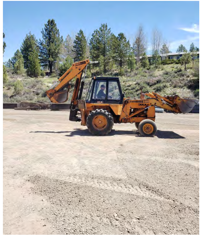
Bart and David Hansen surfacing the parking lot with fresh road base.
