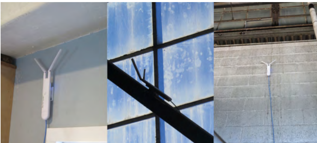
New Museum WiFi installed by Kenneth Finnegan & Kerry Cochran. Access points are now in the Silver Debris (crew lounge), southwest corner of diesel shop and near the Museum Store - photos by Kerry Cochran
