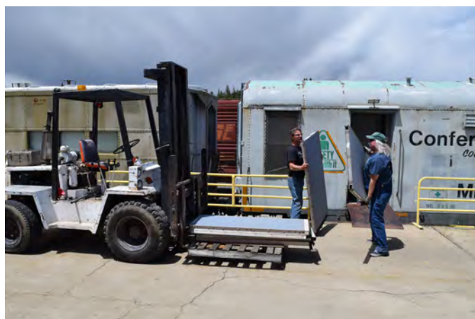
Vince Bonfiglio and Phil Schmierer helping remove partitions from the Archive Car to be moved to another archive department boxcar. - photo by Ethan Doty
