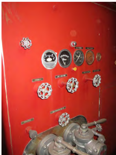
Controls and under the hood of the fire truck
