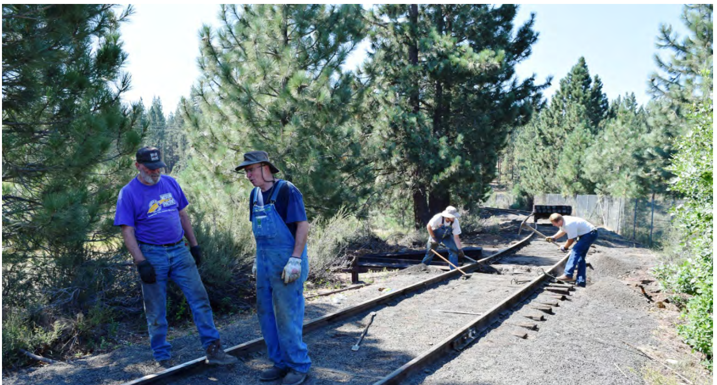
Bil Jackson and Roger Stabler discuss tamping needs on 9 August 2017 as Ethan Doty and Jason Peterich prepare the next tie insert location. Roger has repaired the tamper and has 6 of the 8 tamper motors working and two motors to install at a later date.
