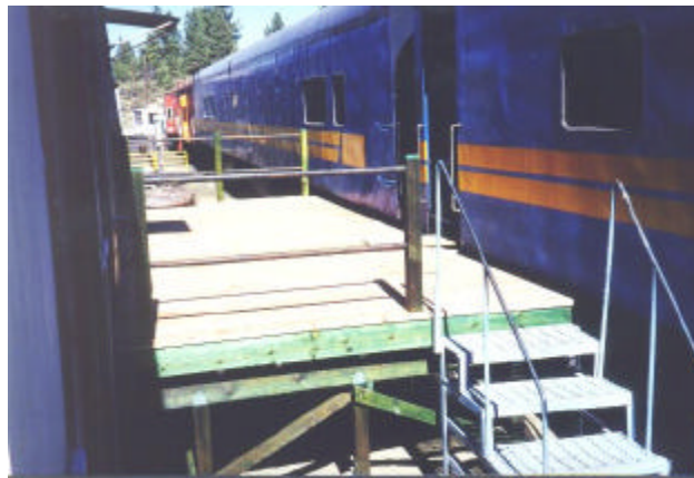
Now complete the new deck between the sleeper and shower car provides a walkway between the two cars as well as a place to bar-b-que lunch or dinner for our volunteers. - Norman Holmes
