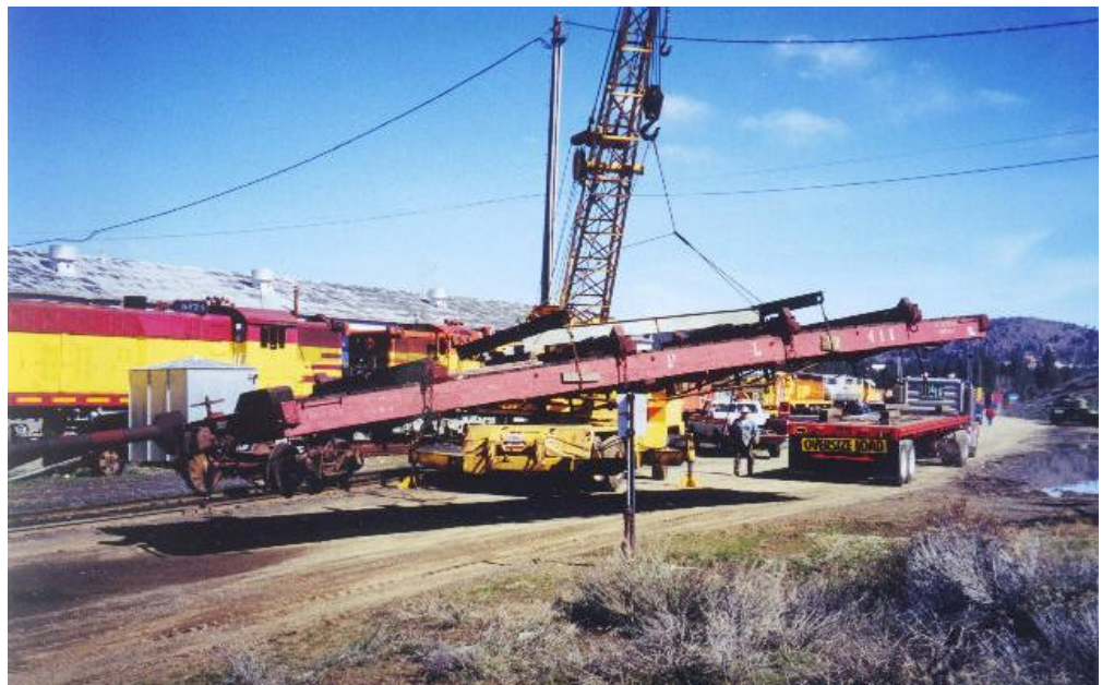
After being lifted from the truck trailer one of the flat cars is being swung around in preparation for setting it back on its arch-bar trucks.
