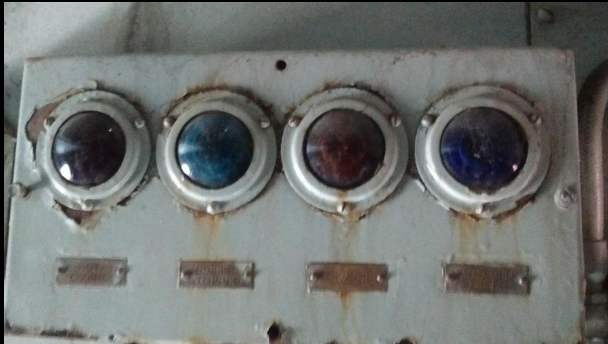
Hot Engine, Boiler Stopped, Low Oil, Alternator Failure
