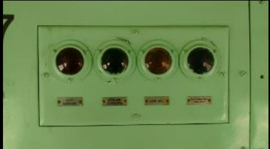
Hot Engine, Boiler Stopped, Low Oil, Alternator Failure
