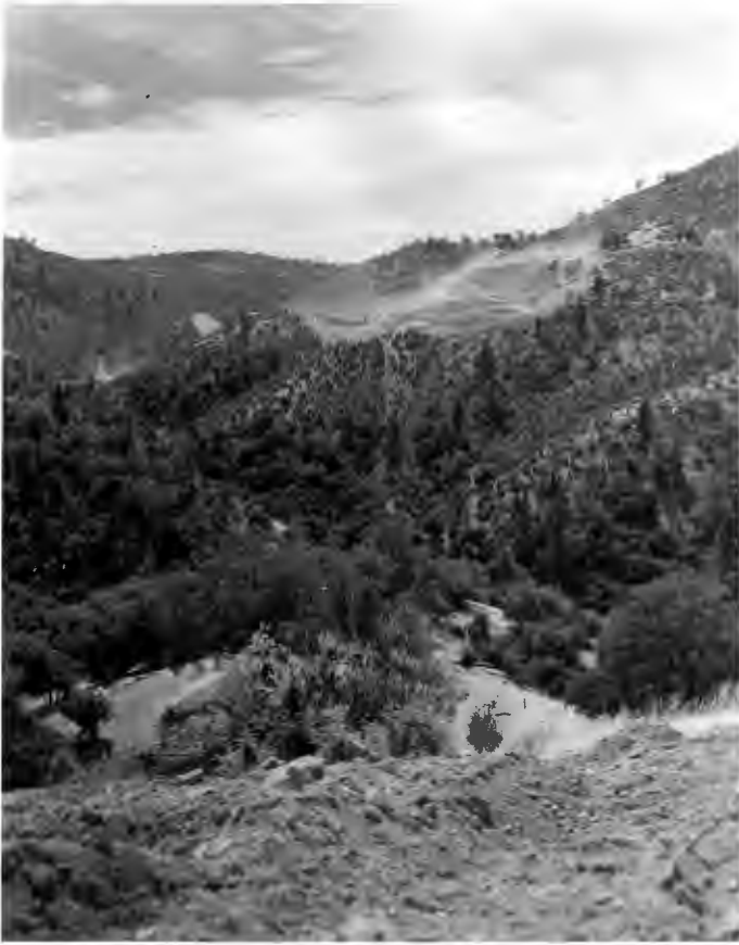
No. 162-1 9-11-58 Wicks Corner - Jarbo Gap Grading operation at the south approach to West Branch Bridge, view from Deer Peak
