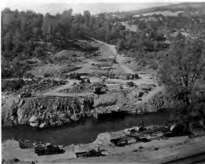
No. 189-4 10-16-58 Feather River Bridge. View ahead on line from Pier No. 2. Crane placing concrete at Pier No. 4.
