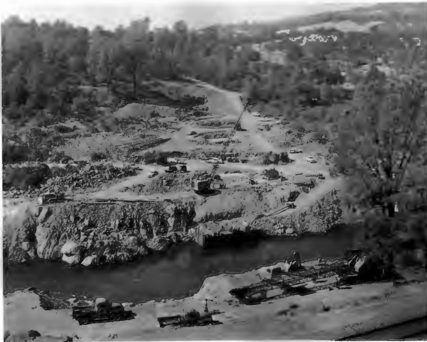
No. 189-4 10-16-58 Feather River Bridge. View ahead on line from Pier No. 2. Crane placing concrete at Pier No. 4.
