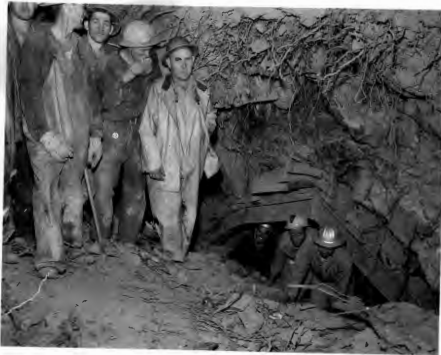
No. 188-3 10-25-58 Tunnel No. 4 (W.P.R.R. No. 7). Hole through at Portal 4 West, 1:44 a.m., October 25, 1958. Ten months elapsed time.
