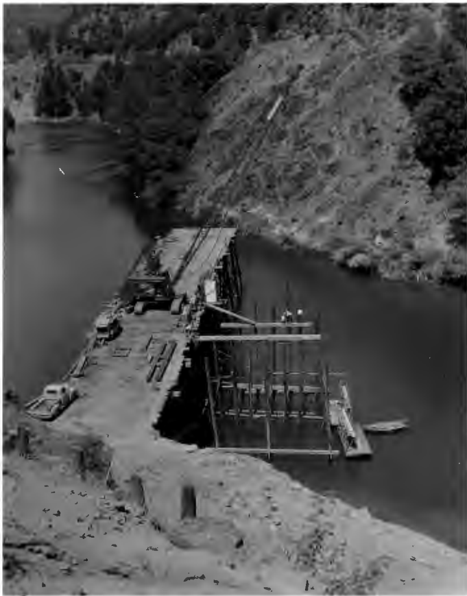
No. 146-5 7-29-58 North Fork Bridge looking upstream at Contractor's work trestle. Pier No. 2 in fore- ground. Pier No. 3 across the river.
