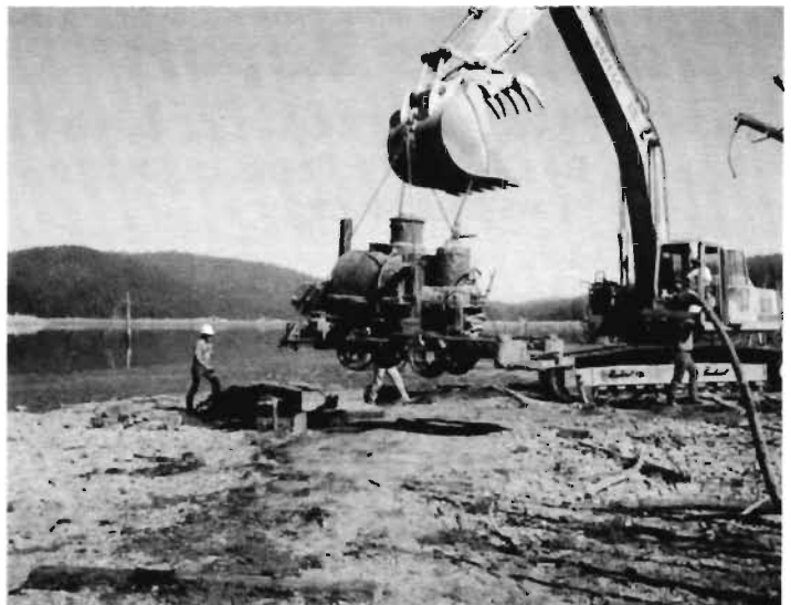
6-ton locomotive is being lifted from its resting place at Butt Lake. Photo by Norm Holmes.
