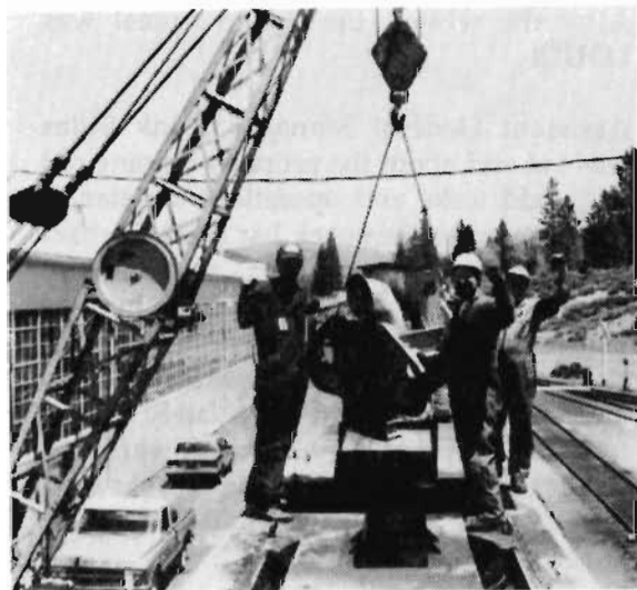
John Ryczkowski, Larry Hanlon and Dave McClain on top of UP 849 (GP-30) as the turbo is removed for repair. (DW)
