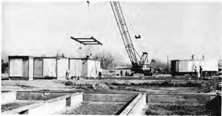
Workers uncouple crane lifting rack from module just placed on foundation, as men ready another module on truck at right for fast transfer to erection site. Up to 20 modules can be placed in position each day.
