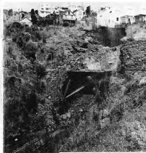
Picture of the south end of Tunnel "A" taken on July 2, two days following outbreak of fire. Portal is nearly filled with rock from slide.
