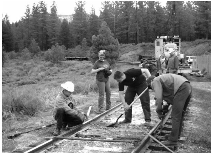
With the 'elder' supervisors observing, our younger volunteers for the weekend assisted with the many repairs to the ballon track.
